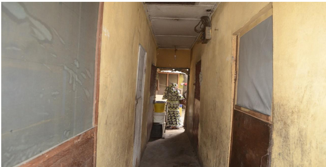
Plate 2. A picture of a typical narrow corridor of tenement houses (face me i face you) in Diobu, Port Harcourt Photo credit. Alagbogu, Gloria Ifeyinwa, 19 th April 2017
